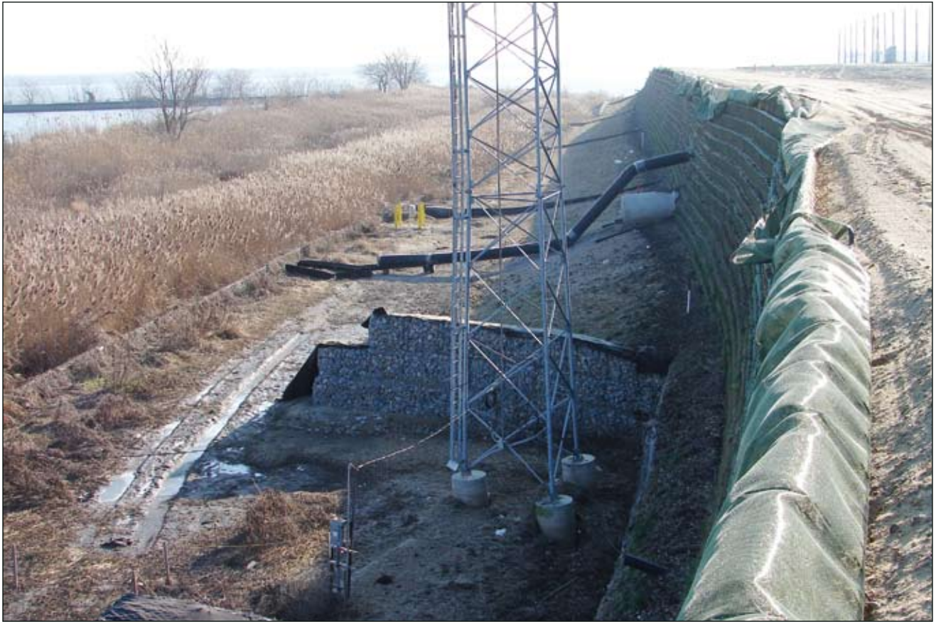
Figure 3. Stormwater management outlet through MSE wall at Cherry Island Landfill.
