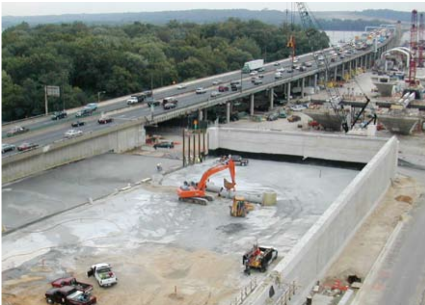
Figure 1. Low density cementitious fill at west approach of Wilson Bridge abutment.
