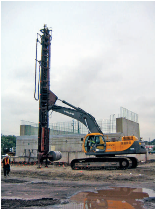
Menard installed 9,000 Prefabricated Vertical Drains (Wick Drains) to depths of up to 30 feet.
